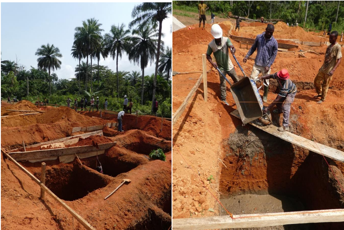
33 large holes (2x2x2m 3 ) were dug by hand for the foundation pillars (Left). Each hole then had a base of cement and block rock as a basis for the pillars (Right).
