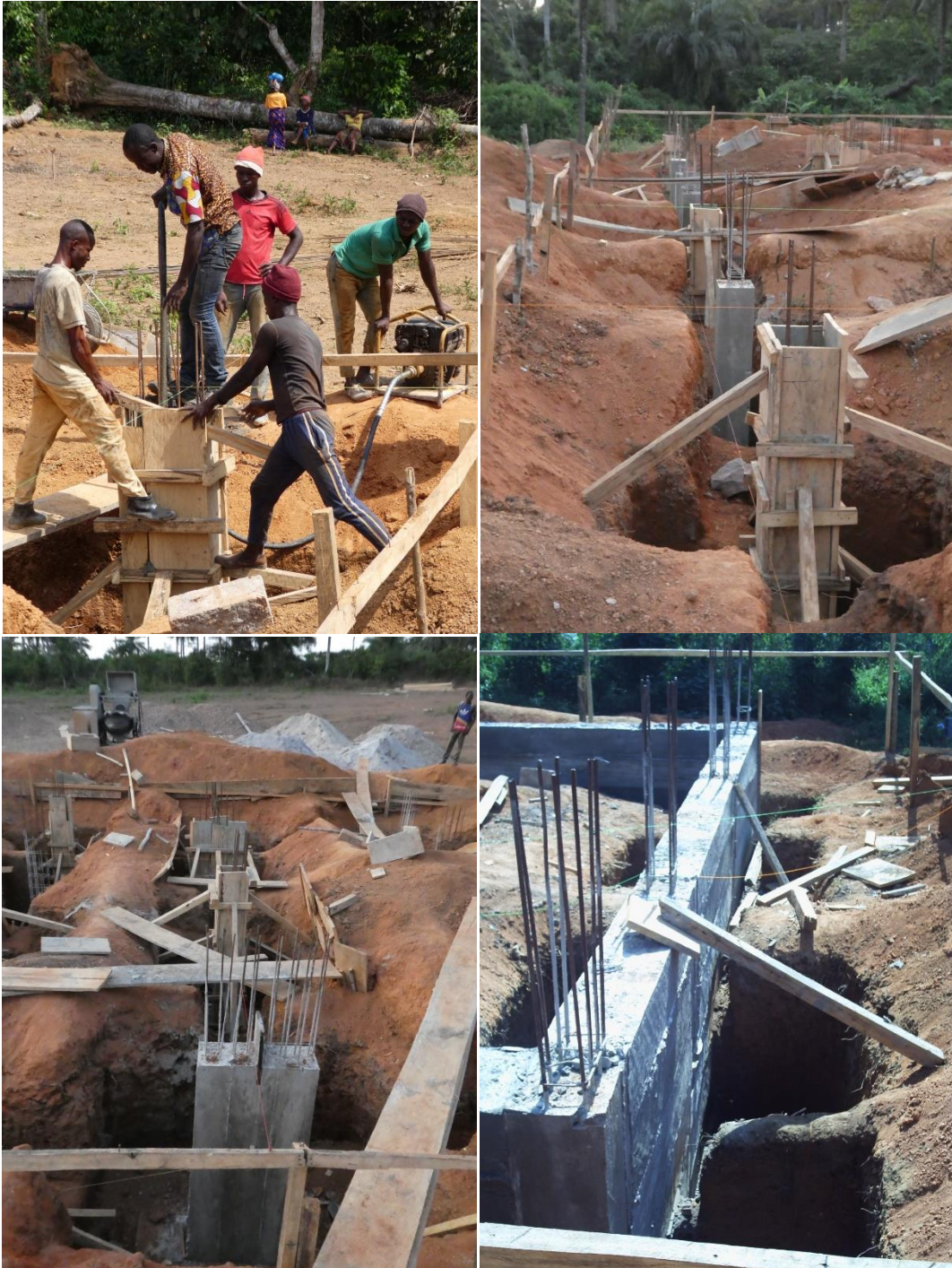
A cement vibrator was hired to ensure the foundation pillars were strong. Once complete the timber framing was removed and the vertical pillars were linked horizontally with more cement to a depth of one metre. The first floor bricks will be built on top of this cement framework.
